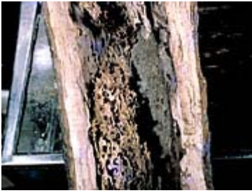
Carpenter Ant damage
