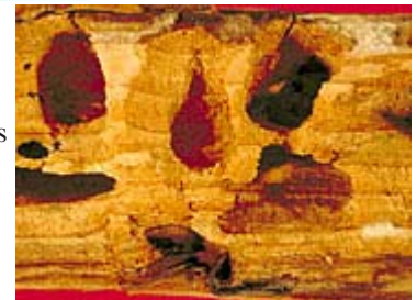
Carpenter Ant galleries (close up)
